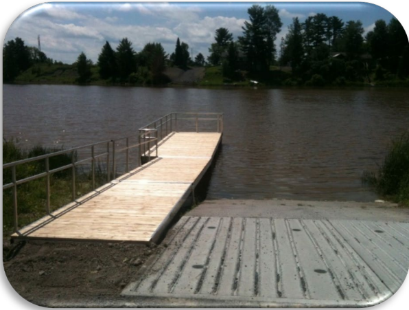
Dock installed at Jessup's Falls Conservation Area with support from fundraising revenue.
