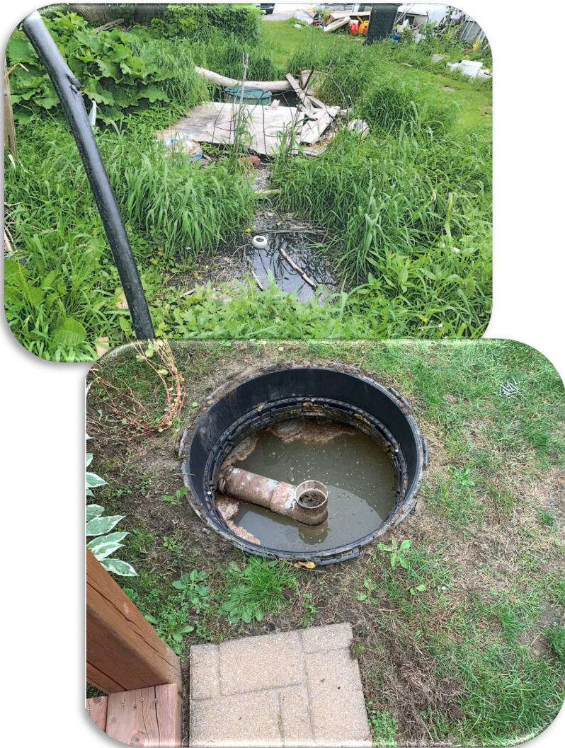
Failed Septic System Discharge
