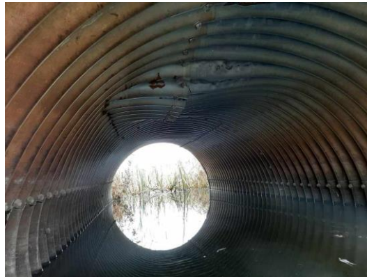
Fig 1: Damage to Culvert
