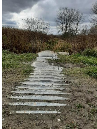
Fig 2: Cover Over Damaged culvert
